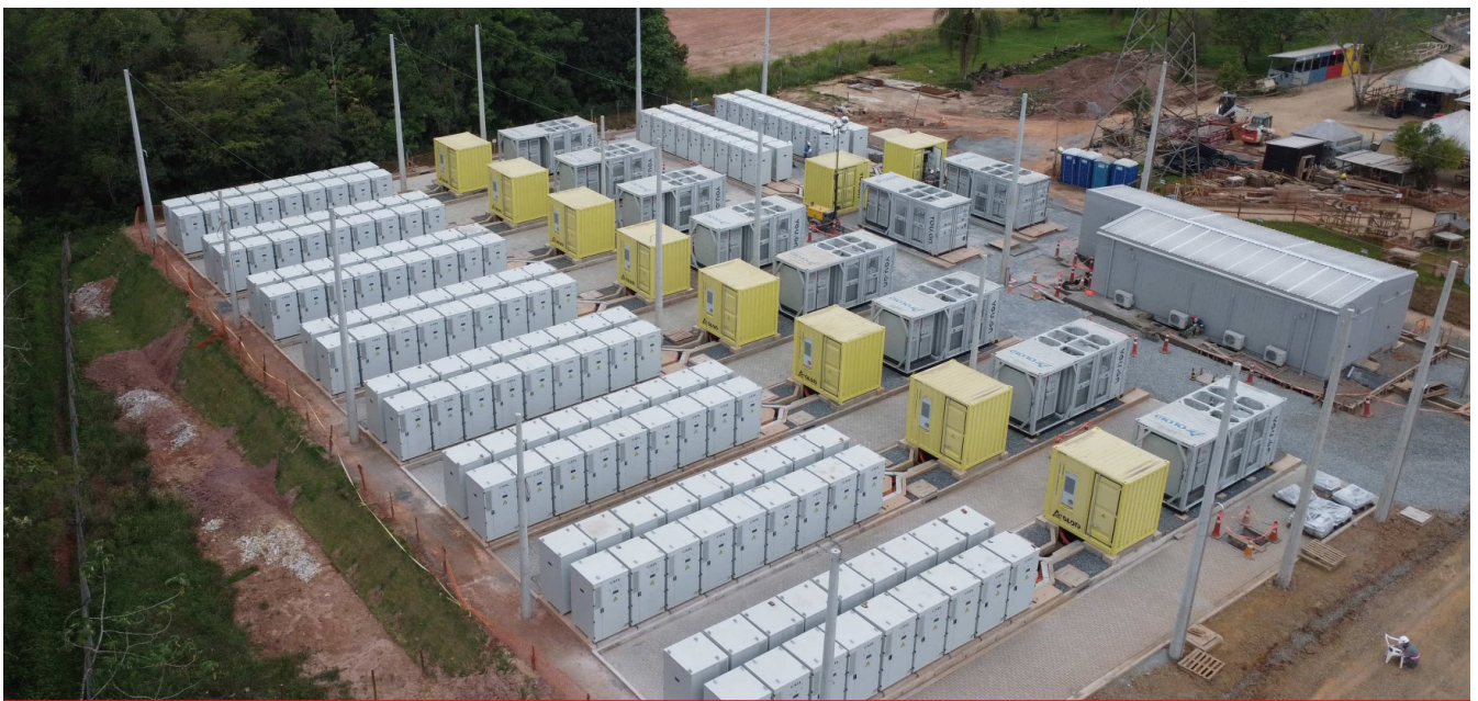
33.5 MW/67 MWh Large-scale Energy Storage Project in Brazil Brazil's largest energy storage project
