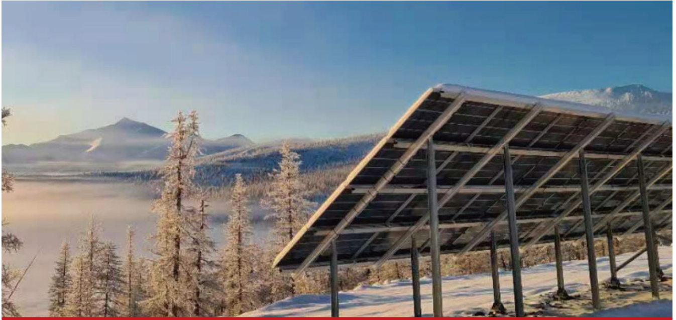
1 MW Energy Storage Project in Europe Located deep in the mountain
