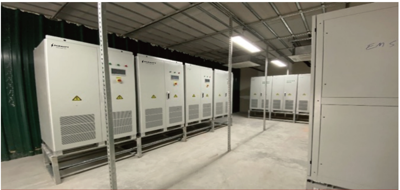
10MW Energy Storage Application in Bahamas
