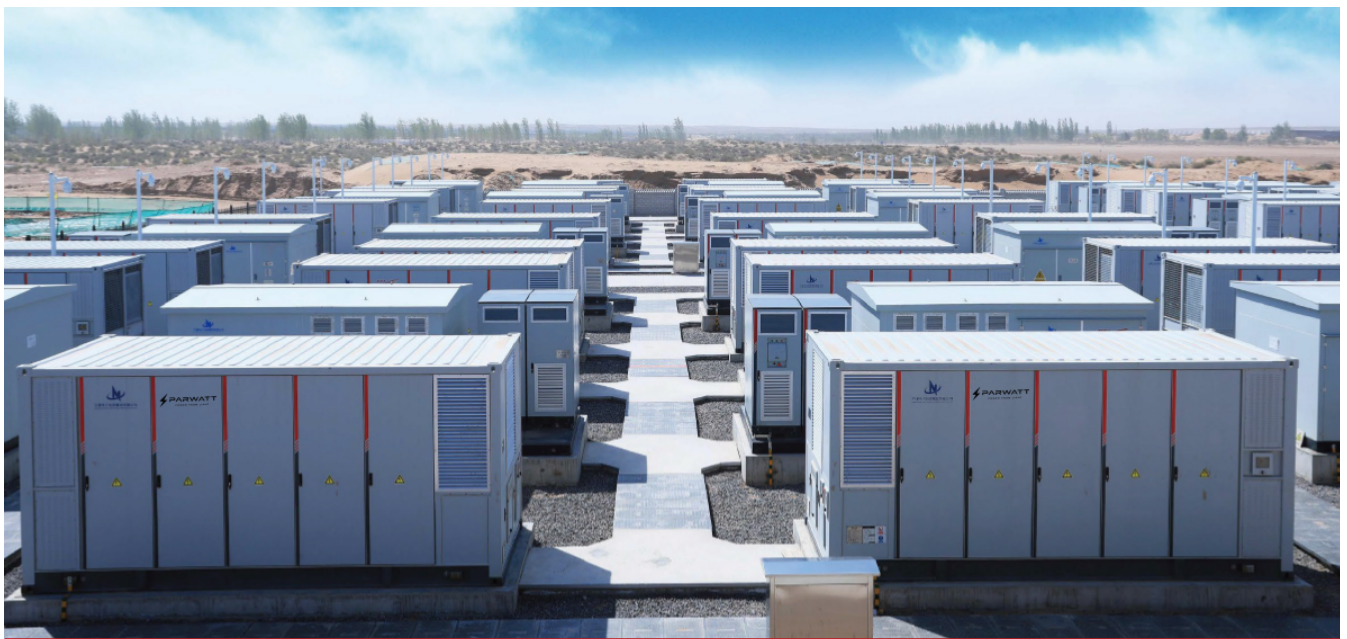
100 MW/200 MWh Co-Located Energy Storage Station in Ningdong Town, Ningxia Hui Autonomous Region
