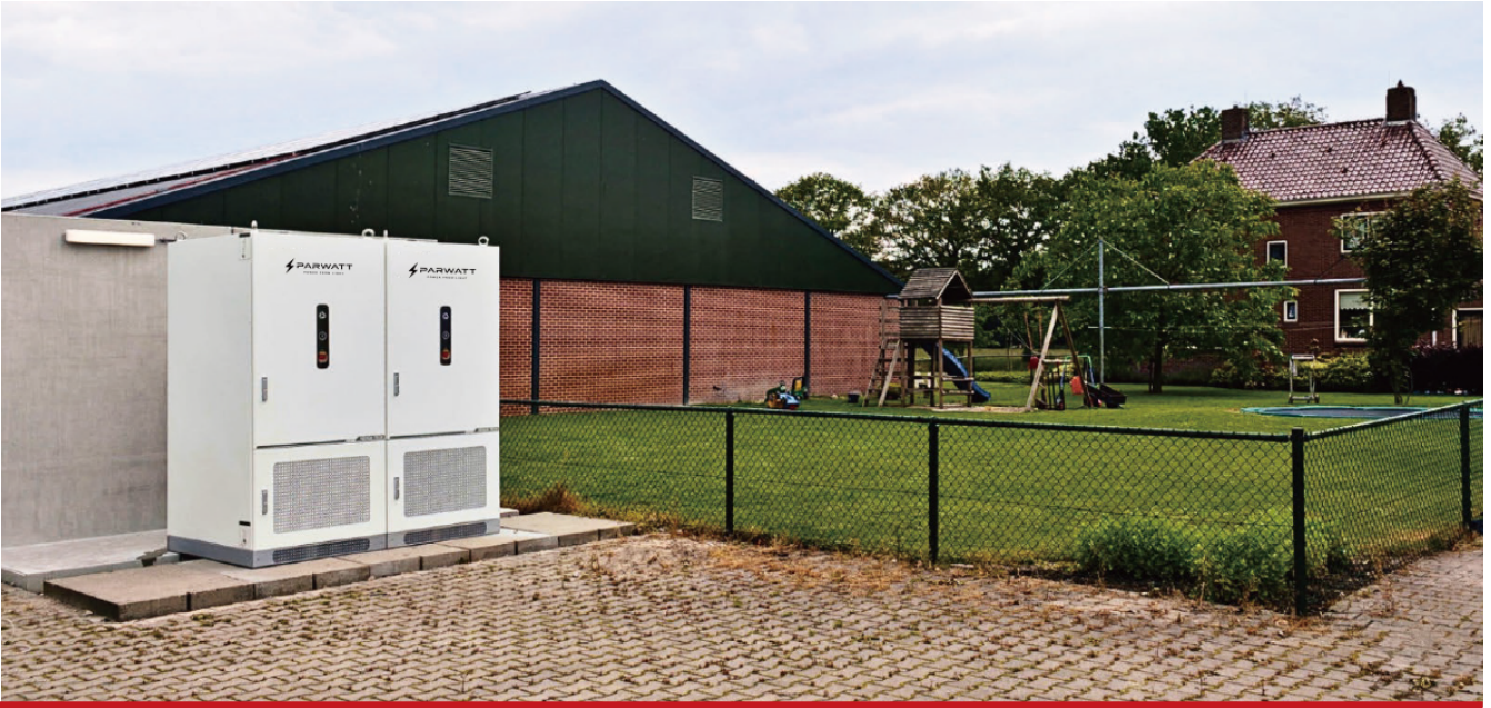
C&I PV+ESS Solution in Netherlands
