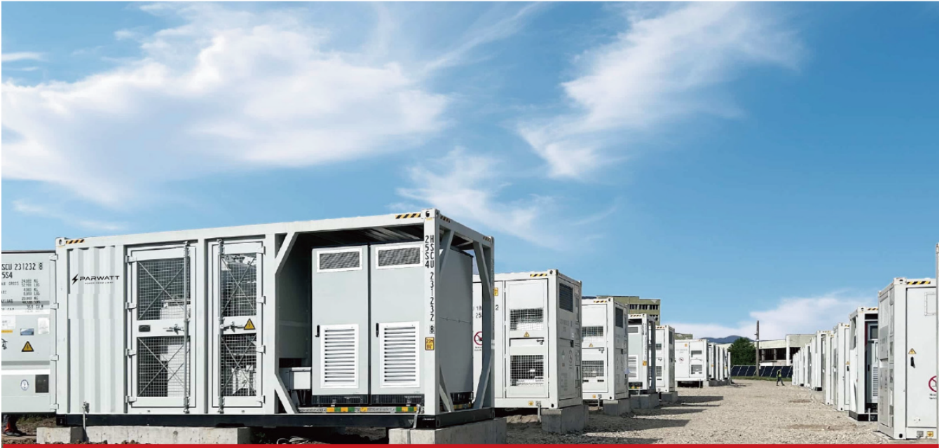
27.6 MW/55 MWh Energy Storage Project in Bulgaria By 2024, Bulgaria's largest energy storage project
