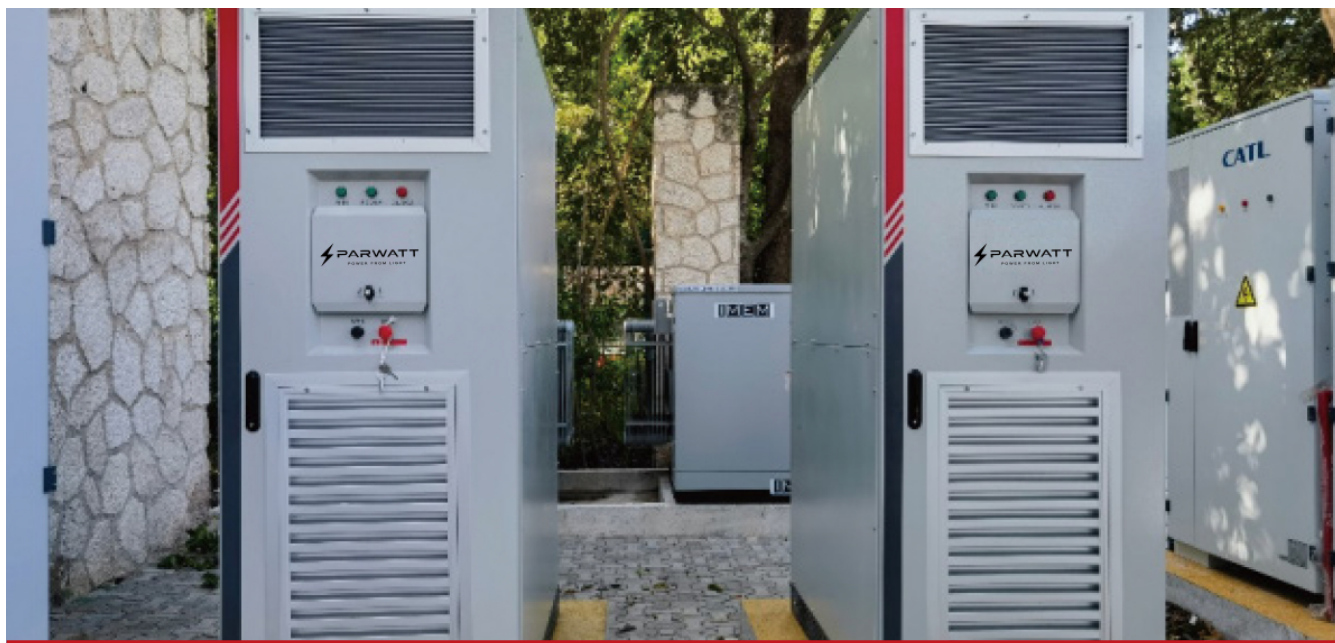
10 MWh C&I Energy Storage Project in Mexico
